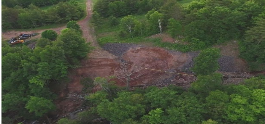
Mont Ripley Landslide following Father's Day Flood
