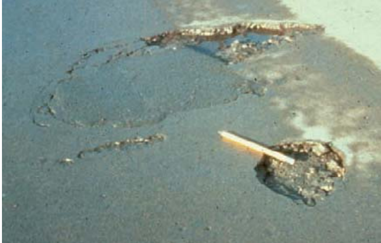
Figure 6: Concrete deck surface scaling (FHWA 2006)
