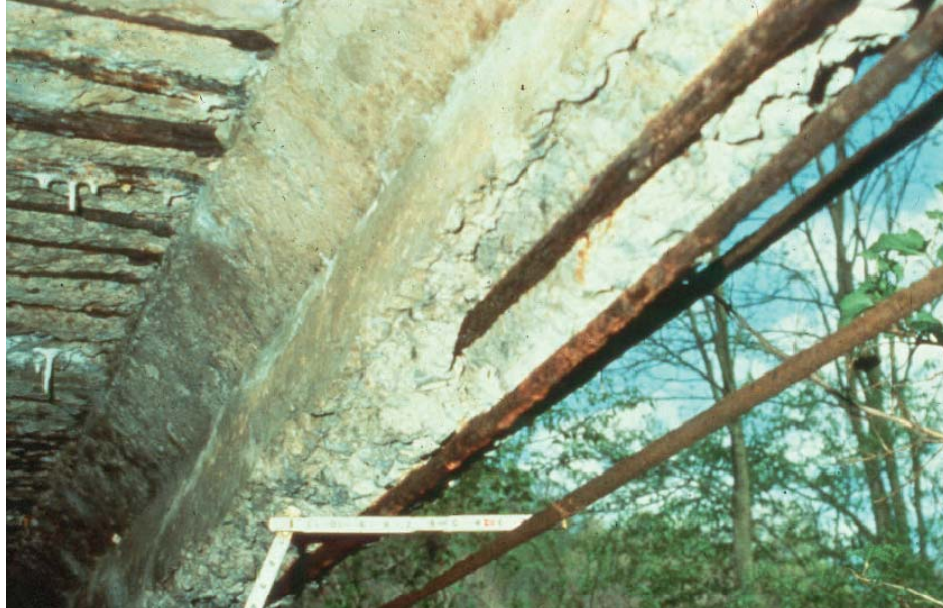
Figure 14: Corroded reinforcing bars
