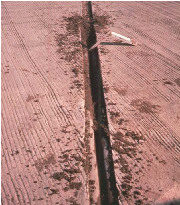
Figure 8: Material in expansion joint (FHWA 2006)
