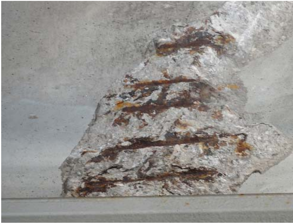
Figure 10: Corroded reinforcement in bridge deck
