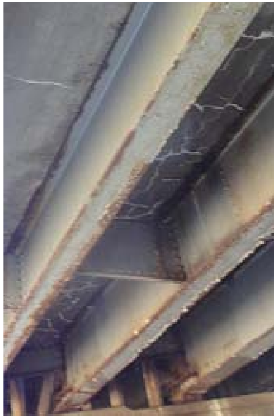
Figure 12: Paint loss on girder surface
