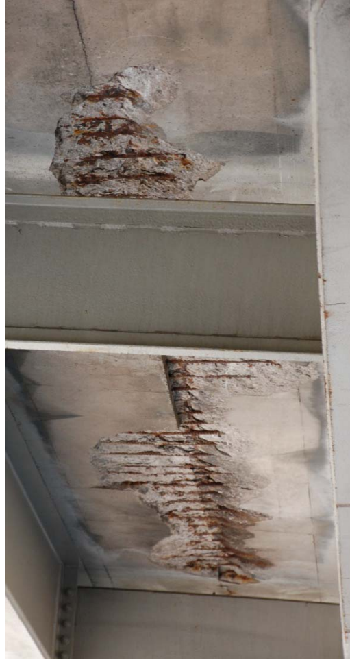
Figure 15: Significant spalling of a bridge bay that merits full replacement
