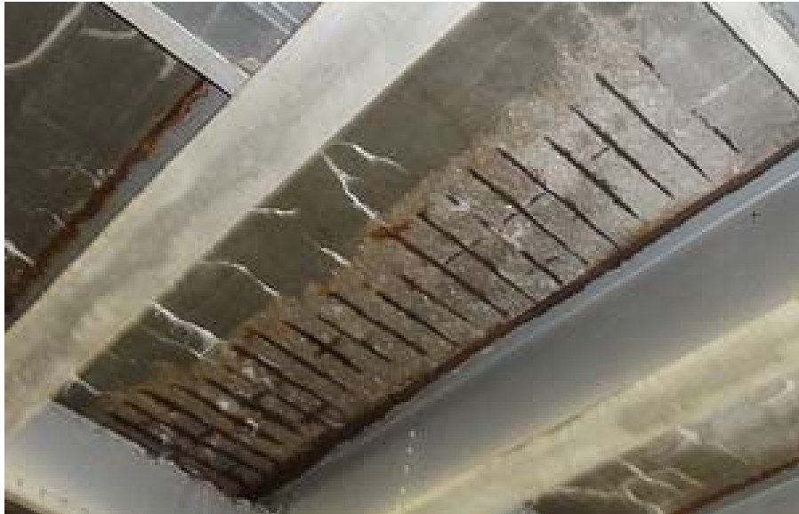
Figure 9: Spalling on bridge deck surface
