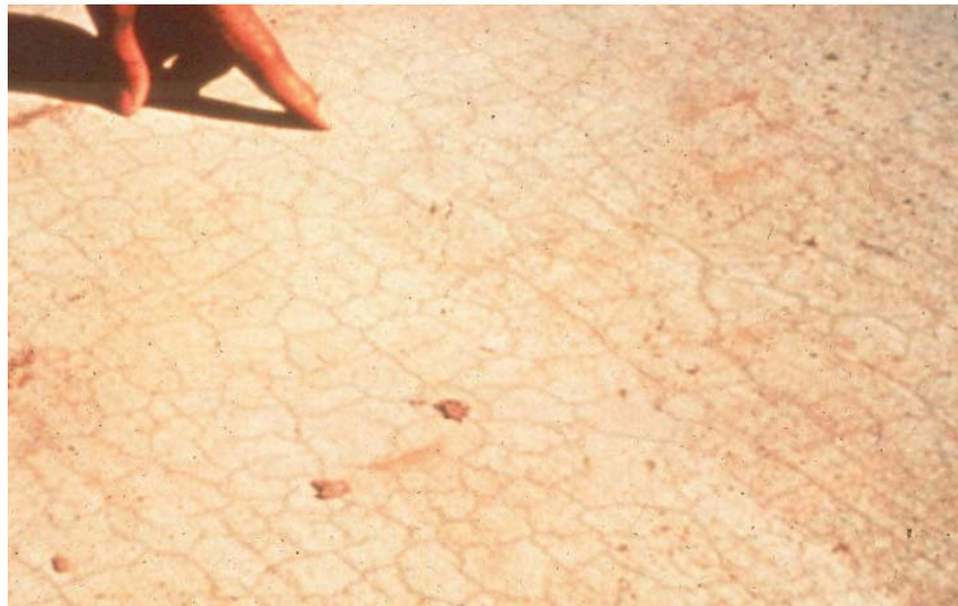
Figure 5: Map cracking on bridge deck surface (FHWA 2006)
