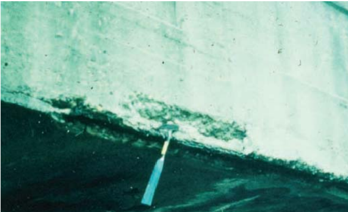
Figure 13: Concrete section loss (FHWA 2006)
